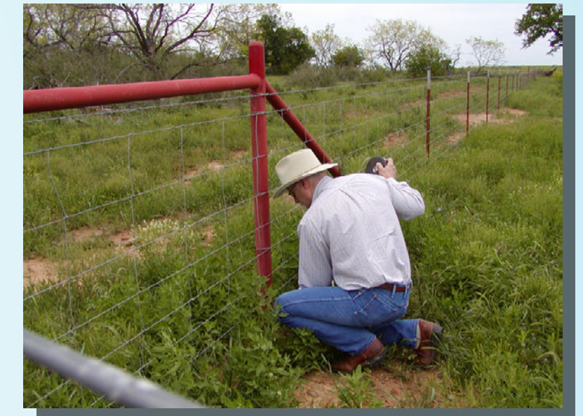
NRCS District Conservationist, Mike Shomette checks progress of cross fence installation through LCRA Creekside Conservation Program.
